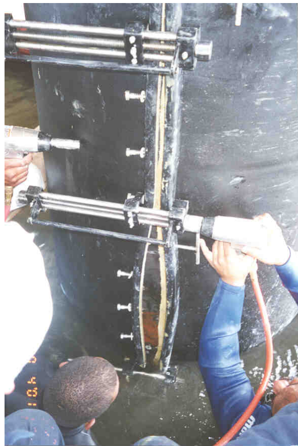
Factory fitted \frac{1}{2} " 316L lag fasteners being driven by impact wrench. Note closure calipers that are used in place of draw bolts.
