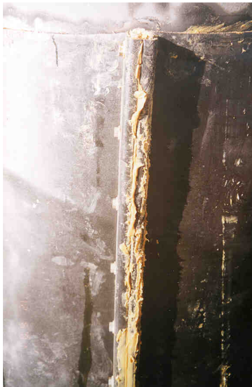
Closure flange showing excess gel exuding after final closure due to residual hoop tension created within wrap fabric.
