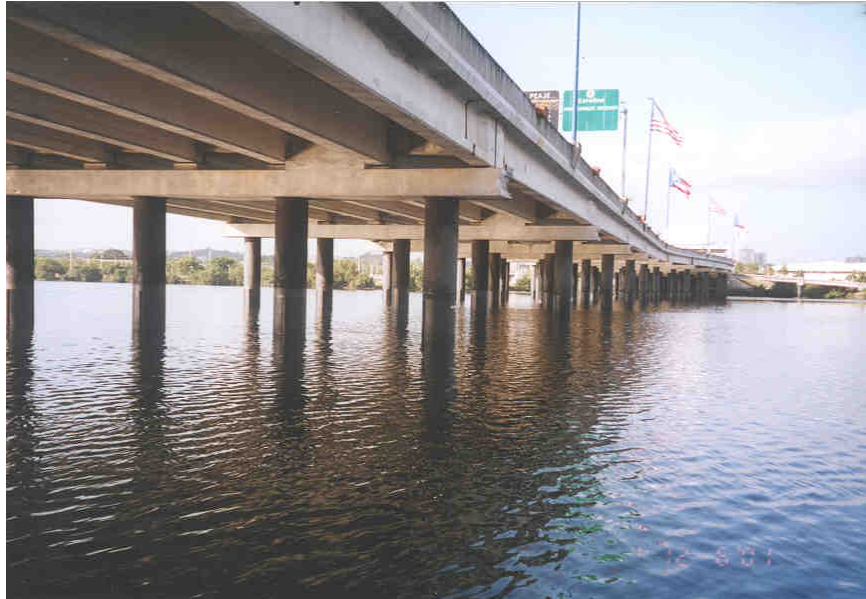
Moscoso Bridge with wraps installed. Toll station end showing density of piles under toll plaza and private access ramp.
