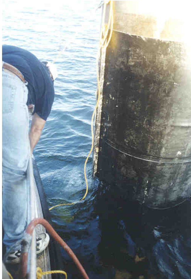
Upper section closure complete with draw bolts removed and permanent fasteners in position. Diver still working below.
