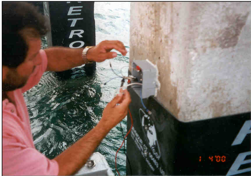
Anode connection terminates within junction box along with output potential monitoring facility.
