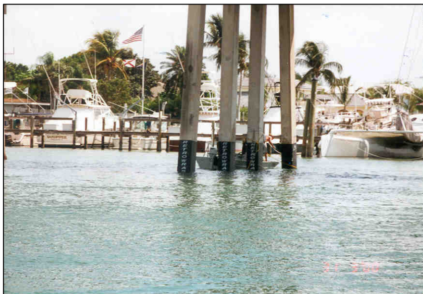
Completed Retrofit installation. Fast, light weight, and esthetically pleasing to the eye.
