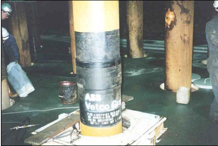
Vetco SR20 connector at work station awaiting installation of low profile SL type wrap.
