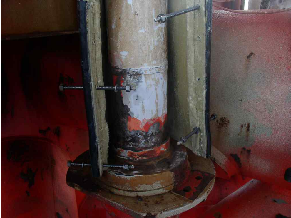
Dual diameter 244/219 transition unit has been lowered onto dead weight support flange. Note: Draw bolts pre fitted into closure flange.
