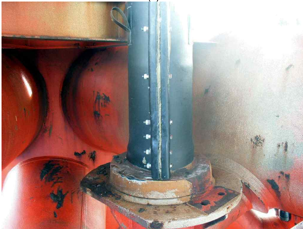
Dual diameter transition unit fully installed. Factory thermal formed flanges visible at neoprene steel interface. Multi bolts at high stress area.
